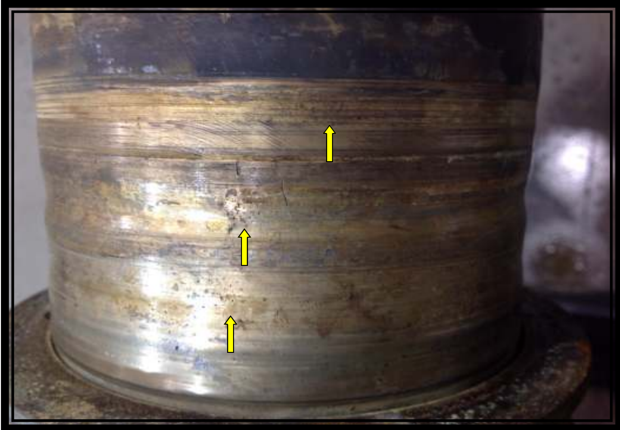
Photo 2: #2 High Service Pump - Bronze Packing Sleeve Pitting and Scoring
