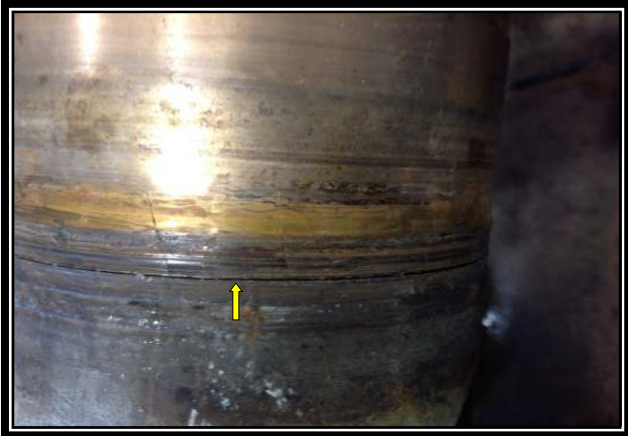
Photo 4: #2 High Service Pump - Bronze Packing Sleeve Full Depth Radial Crack
