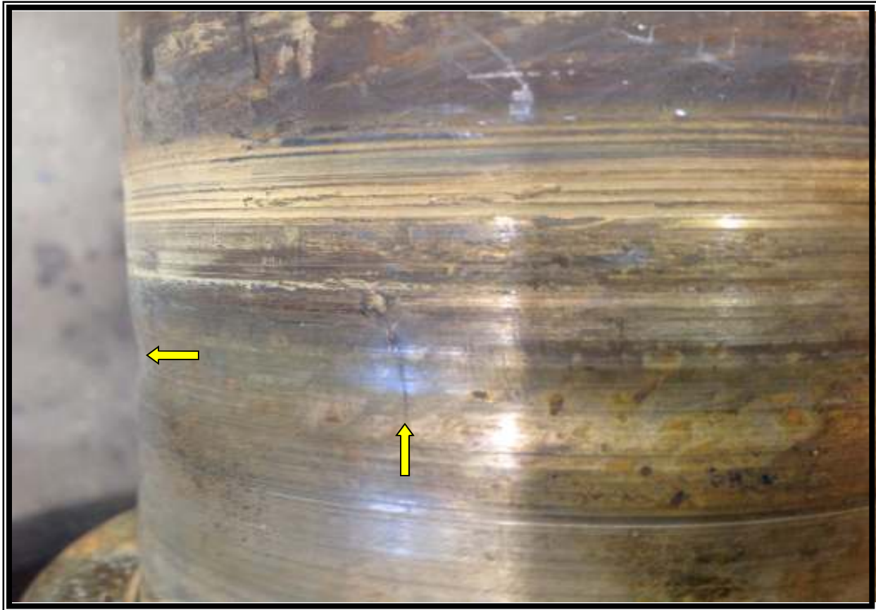
Photo 3 : #2 High Service Pump - Bronze Packing Sleeve Wear Grooves & Cracks
