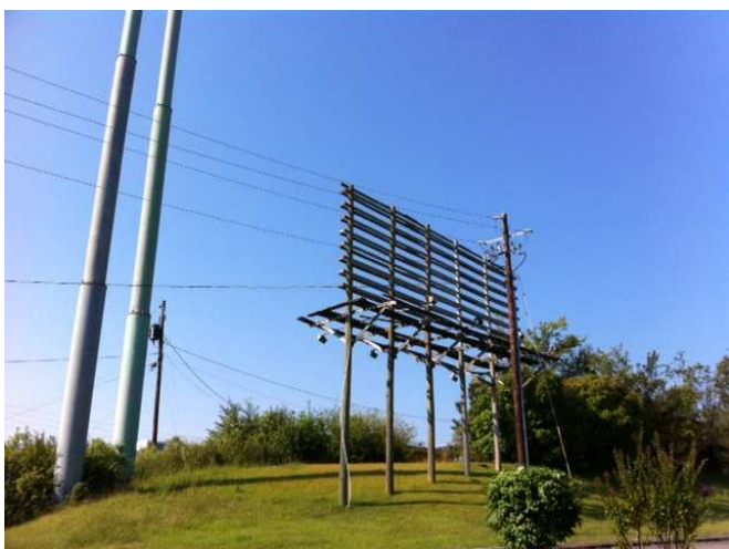
This area includes dilapidated and unused billboards.
