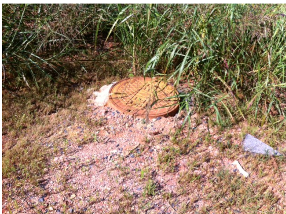
This area contains deteriorating infrastructure.
